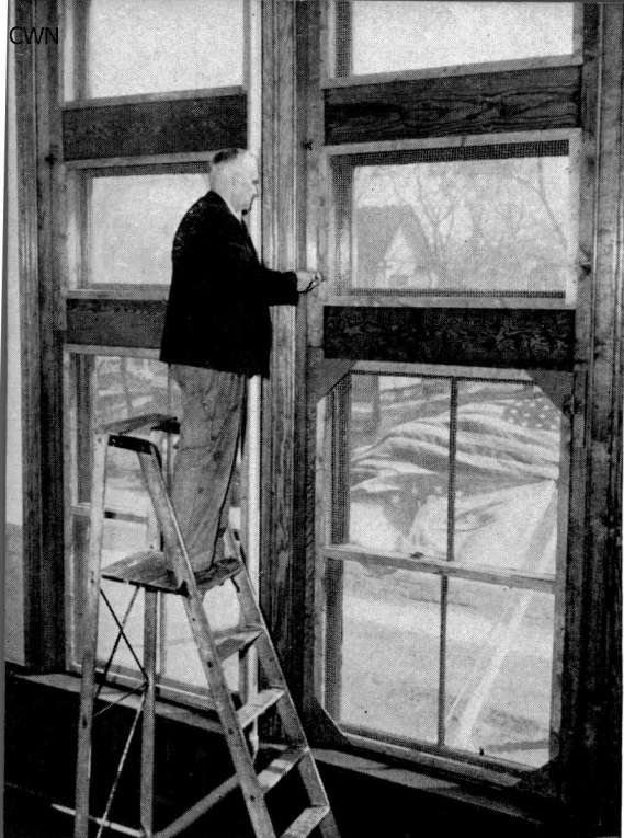
Rupert Cady, a City carpenter, installs a wire mesh screen to protect children of Rice School from flying glass in event of an air raid.
